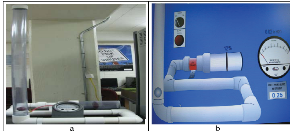
Figure 2.16 The Industrial Blower Control System
